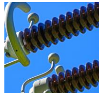
Substation and Grid Components
