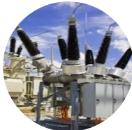
Substation and Grid Components
