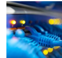
Network Infrastructure and Security
